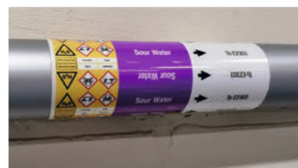
Pipe Marking according ISO 20560-1
